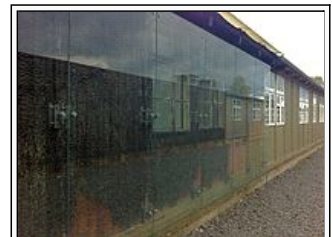
Arson damage caused to this barrack building has been covered in glass to protect it, whilst still showing the damage to those visiting the camp.
